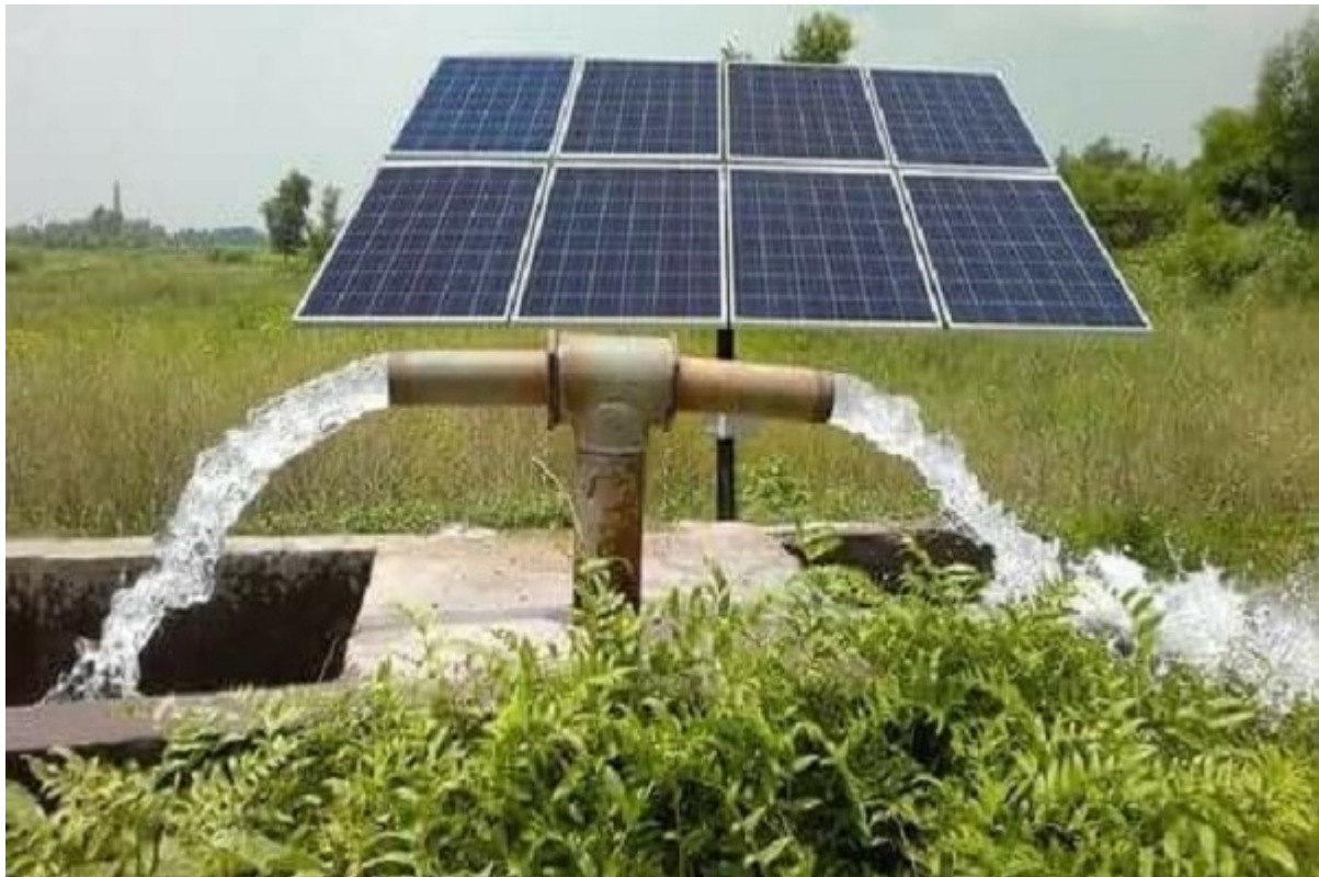
A view of solar pump
